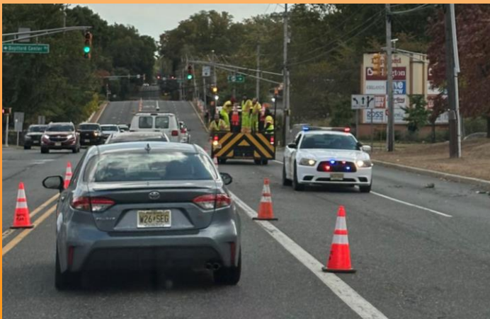
Nothing here will provide protection to the workers on the back of the cone truck.
